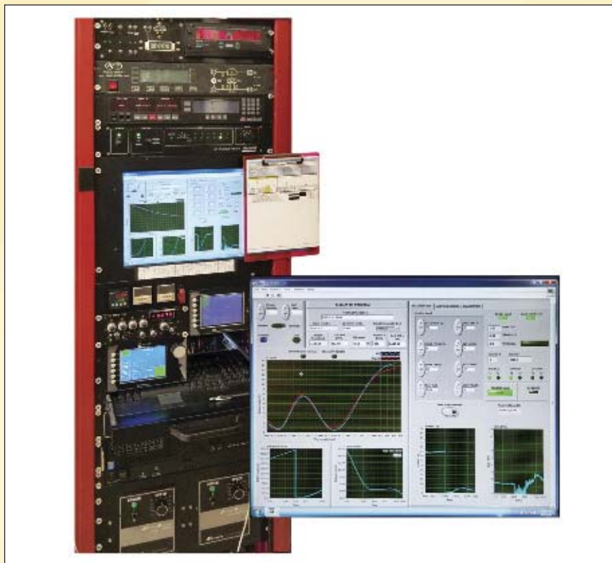
Figure 4. SpectraLock Controller and IDEM software screen capture during monitoring process.
